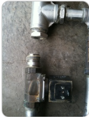
Step 6: Remove valve Remove the bad solenoid valve from the plumbing assembly
